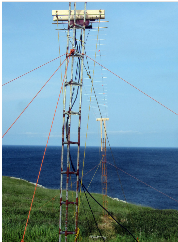
Figure 6: Ultra-light yagi operating in transatlantic service at Pouch Cove, Newfoundland. Notice the adjustable wood top section on the front tower, compensating for ground slope, and the use of five guys per tower to allow substantial tension to be applied to the Kevlar booms. The forward guy ropes on the front tower attach to the steel eye-bolts holding the tower pulley block in place, so the antenna exerts its pull on the eye-bolts and guys, not the wooden leg extensions. The rear tower's two forward legs are not exactly 90° to the yagi's long axis, easily compensated for by adjusting the right and left side antenna-tensioning halyards. The pulley pairs at the feedpoint are locked together so that the weight of the cables, preamplifier, driven element and so on won't cause sway or sag. Tension adjustments are made at the forward end, where there the two wood pulley blocks are several feet apart. We used "seasoned" steel TV towers from a Newfoundland forest, thanks to Joe, VO1NA!
