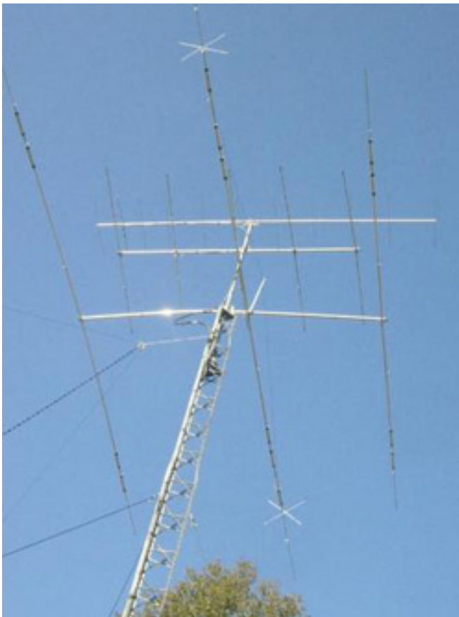
The antennas at WK4P. The tribander and wire did all the work this time. (Photo – WK4P)
