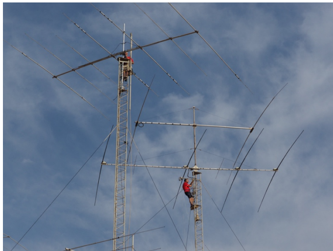
W2GD (left) and DL6RAI (right) performing tower work at P49V in Aruba during the week before the contest. The work was finished just in time for DH8BQA, DL5CW, DL5LYM, DL6RAI to operate the Multioperator, Two Transmitter P40XM together for the first time. [Oliver Droese, DH8BQA, photo]
