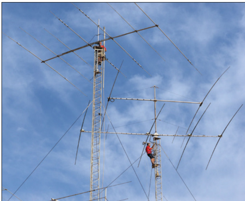
W2GD (left) and DL6RAI (right) performing tower work at P49V in Aruba during the week before the contest. The work was finished just in time for DH8BQA, DL5CW, DL5LYM, and DL6RAI to operate Multioperator, Two Transmitter P40XM together for the first time. [Oliver Droese, DH8BQA, photo]
