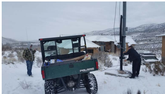
Mike Russo, N6EVG and Heiko Muench, KF7STT try their best for antenna repairs under challenging conditions. (Photo provided by Rick Crockett, WØPC)
