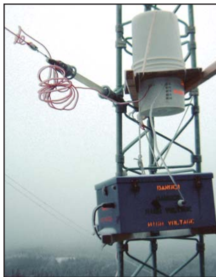
Figure 5—After almost two years of tuning the antenna from inside the shack, in January 2005 VO1NA moved the loading coil and variometer outside to the tower. A smaller variometer, about 60-250 μH, was used in series with a tapped loading coil. This moves the RF and high voltages away from the house. A standard 50 Ω coaxial cable runs back to the transmitter in the shack.
