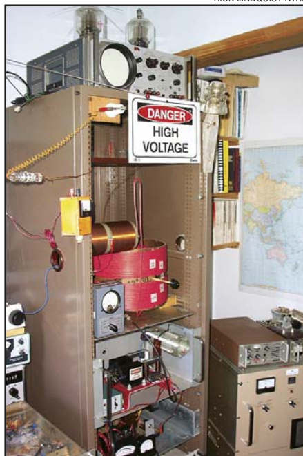
Figure 3—This rack holds the IRF640 power amplifier, power supply, antenna matching coil and variometer for VO1NA’s 137-kHz transmitter. The variometer (L3) is the big red coil on the upper shelf next to the wattmeter. The matching coil (L2) is above the wattmeter. The power amplifier is on the next shelf down (with heat sink, L1, T1 and RFC1). Note that about 2000 V is present at the feedthrough insulator during transmissions.
