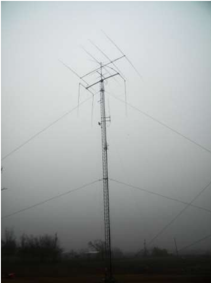
WØUO shunt-fed tower after winter ice storm (WØUO photo)
