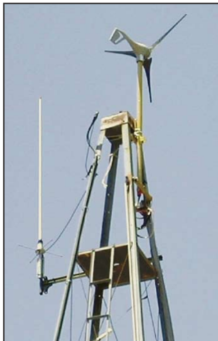
This is the windmill that runs the AB6VS repeater site. With a total cost of under $1000, it not only saves the Loma Prieta Amateur Radio Club money on the electric bill, it saves energy, too.
